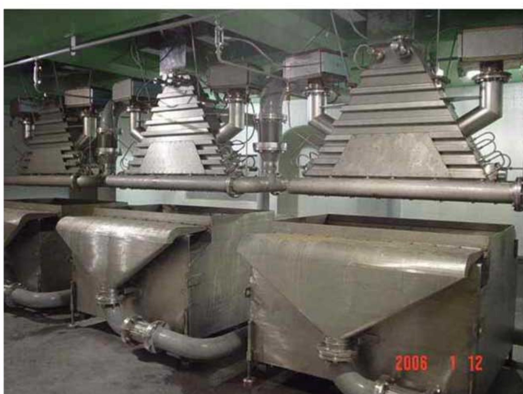
Commercial waste water treatment plant
