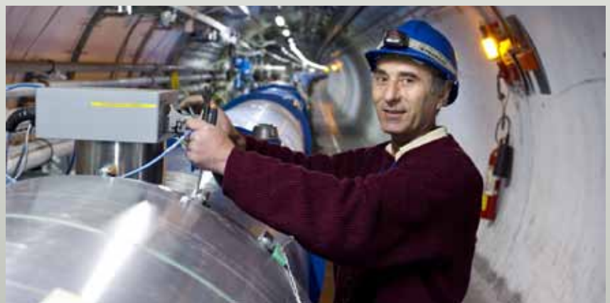
Installing the new Quench Protection System, January 2010. (Credit: CERN)
